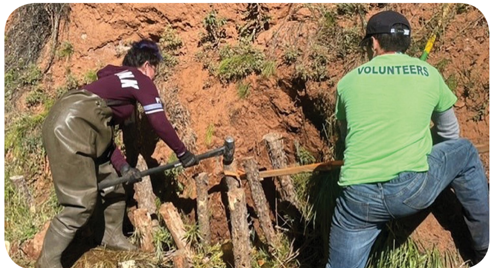
Volunteers pound logs vertically into a streambank in Campbell Valley before weaving willows between them and adding sod. This type of structure forces a stream to meander, rather than going straight downhill and dumping sediment on downstream users. WRV photo, 2022.
