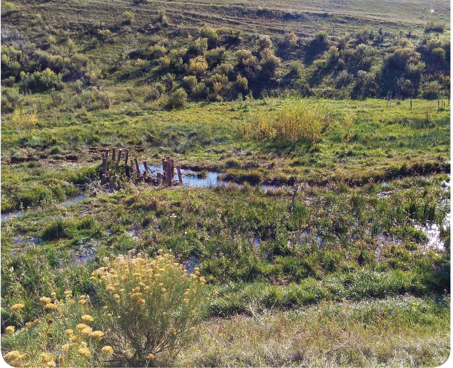
A formerly incised (deeply cut) stream in Campbell Valley where a volunteer-built temporary wooden in-stream structure slows the water, which drops sediment in the surrounding floodplain before moving downriver. Thanks to you and WRV volunteers, this important habitat connection in the Laramie Foothills Mountains to Plains zone now better supports the native wildlife that have evolved here. WRV photo, 2022.
