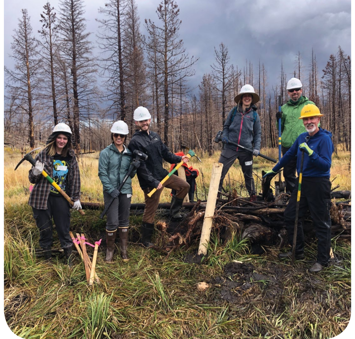
Volunteers and staff pose with an in-stream structure that was built with your funds to reduce risk of flooding and erosion in the Cameron Peak Fire burn scar. WRV photo, 2022.
