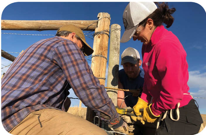
Your support, and that of CDPHE, made it possible for volunteers work together to repair a fence to protect springs, seeps and wetlands from cattle. WRV photo, 2019.
