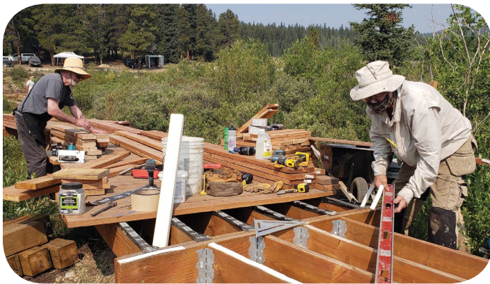
Volunteers prepare a turn in the boardwalk as it snakes between wetland plants. WRV photo, 2021.
